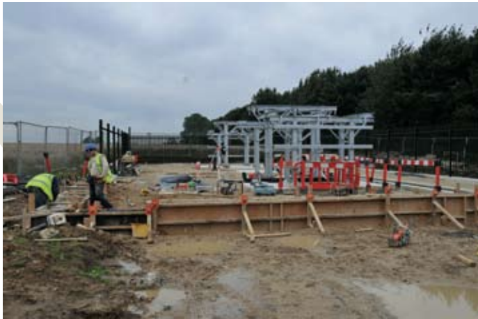
Fig. 2 YEDL HV Compound
