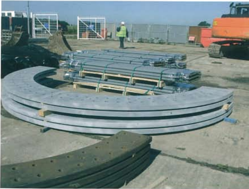
FIG. 3 TURBINE HOLDING-DOWN BOLTS
